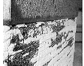
Removal of soft and deteriorated plaster at Prairie Band Polawatomie Indian Nation, KS
